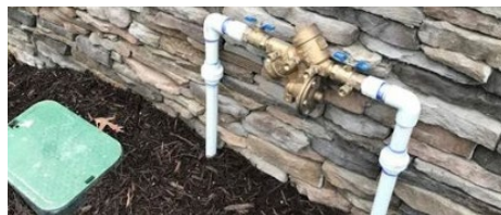
A common example of an RPZ installation
