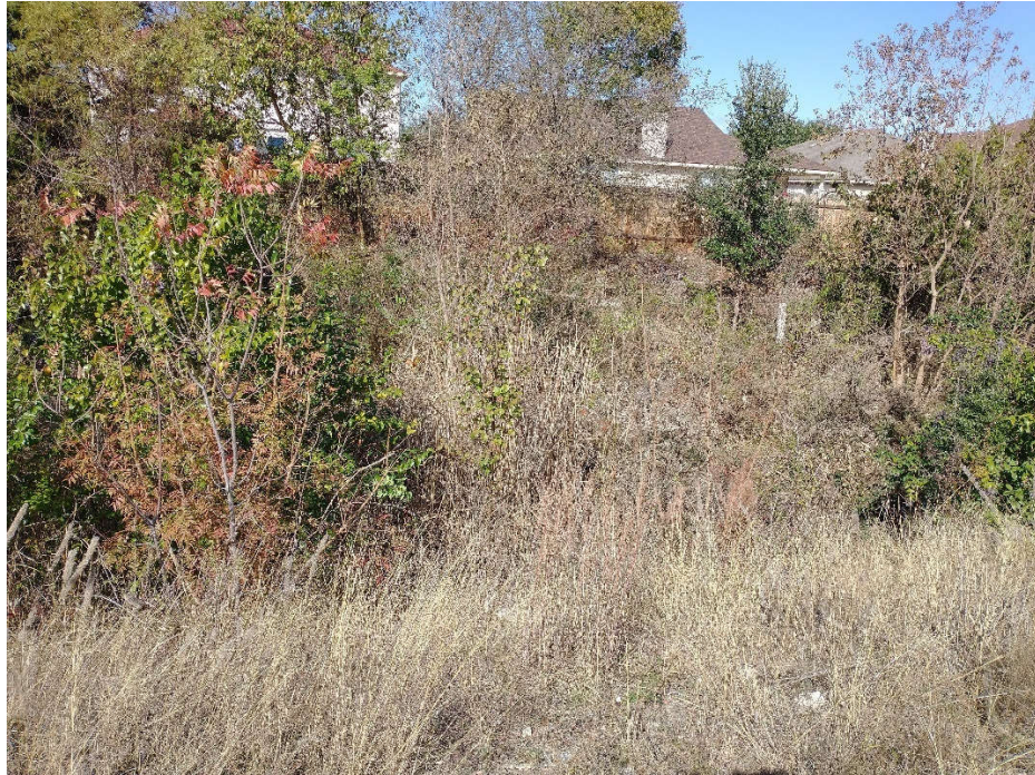
Susan Channel West – Dense vegetation and trees growing in the overbanks of the channel
