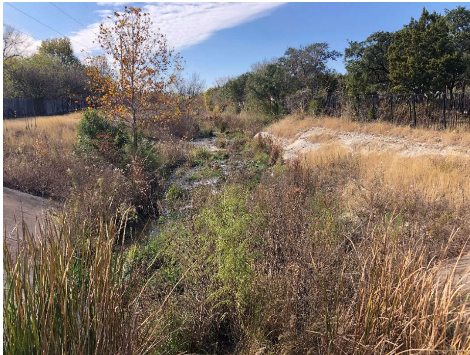
Susan Channel West – Vegetation growing in the channel bed west of Block House Drive
